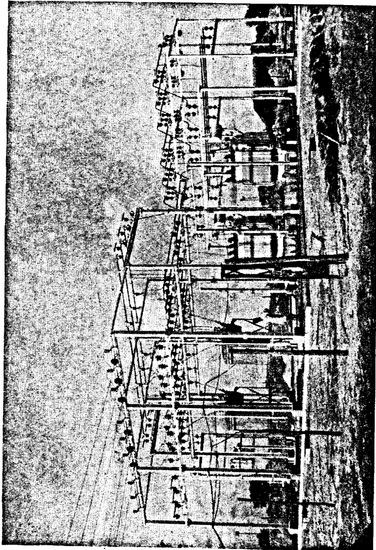
KILANUR—A VIEW OF THE 2 NOS. 1000 KVA. TRANSFORMERS ERECTED AT KILANUR S.S.
