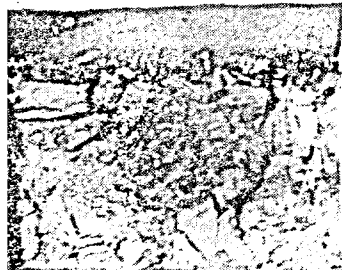
Photo 5. Two coats of surface dressing with stone chips blinding in both coats. Water has penetrated into the base.
